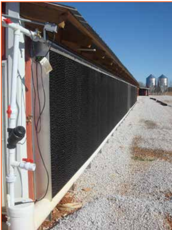
Figure 45: Example of a cooling pad installed on the sidewall of the house (in a 'doghouse').
