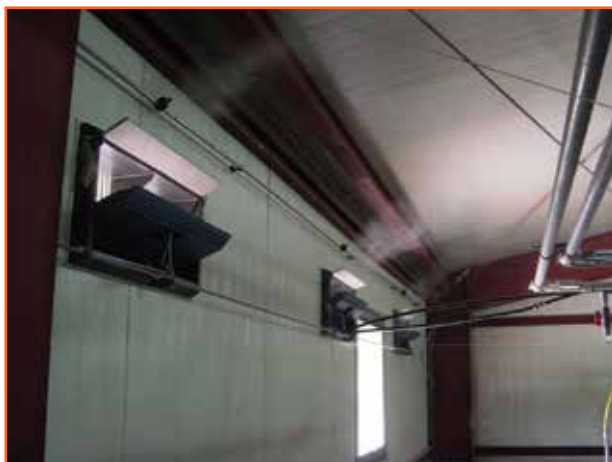
Figure 46: Example fogging system for a cross ventilated house.
