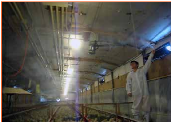
Figure 34: Using a smoke test to determine if airflow and operating pressure is correct.
