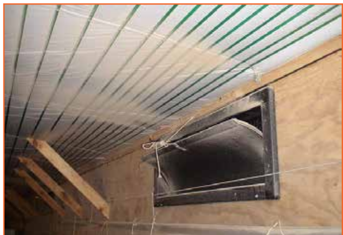
Figure 36: Example of a good quality air inlet.
